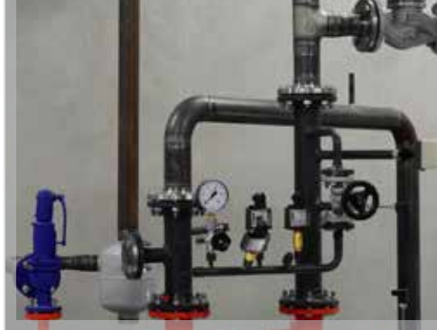
Water Line Pipes
